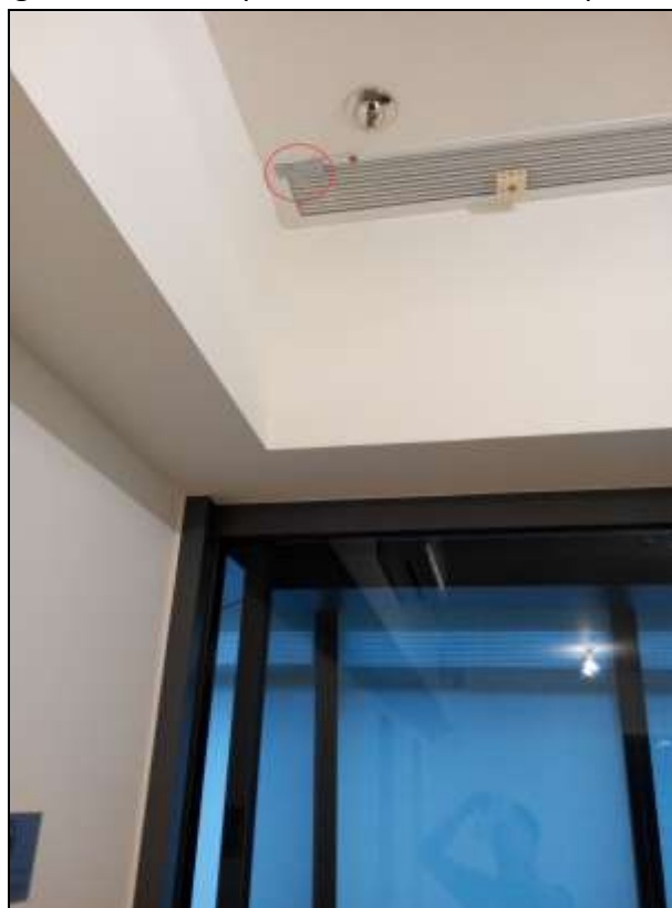
Figure 49: Notice placed in unreasonable position
